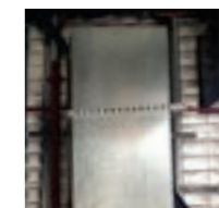
Air Vent and Ducting Reference Officeworks ceiling Photograph taken by Tyler Hill
